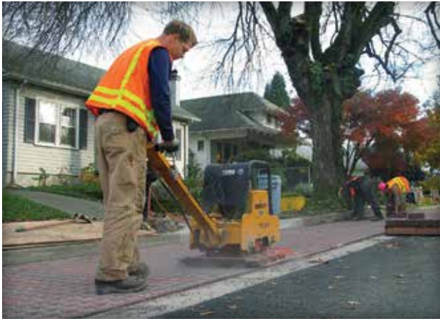
Figure 29. PICP paver compaction shows that pavers need to be set about \frac{3}{4} in. (19 mm) above their final elevation before compaction and \frac{3}{8} in. (10mm) after compaction to account for downward movement.
